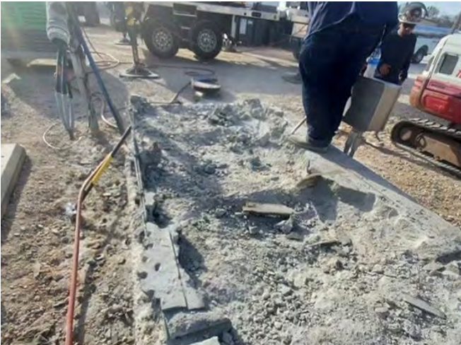
Clear indication of previous epoxy grout had delaminated from the concrete foundation and baseplate. Contractor beginning the demo process
